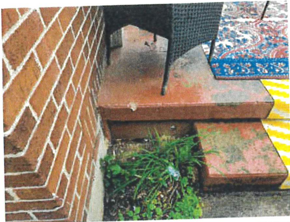
Possible rodent burrow on the side the of the front porch. 5/26/2022 AJL
